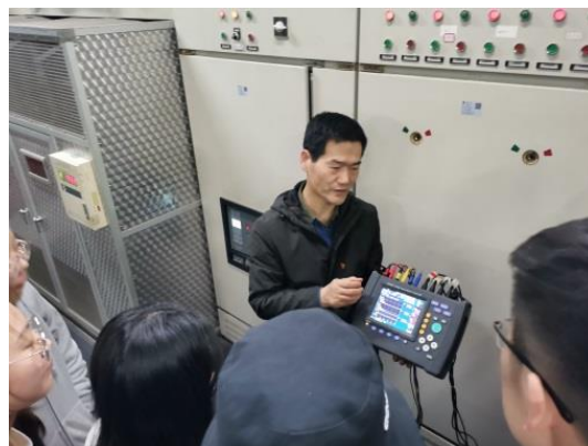
Figure 3. Power quality test in low-voltage distribution substation.
